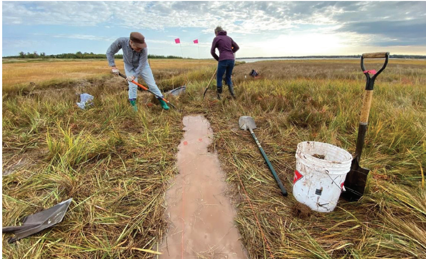
Figure 5. Volunteers digging runnels (shallow ditches) with shovels to drain the surface water off the marsh and restore “proper” hydrology to the site, thus restoring the marsh (taken October 2020). A sill is installed at the mouth of the runnels to slow or halt water flow and reduce the loss of sediment.
