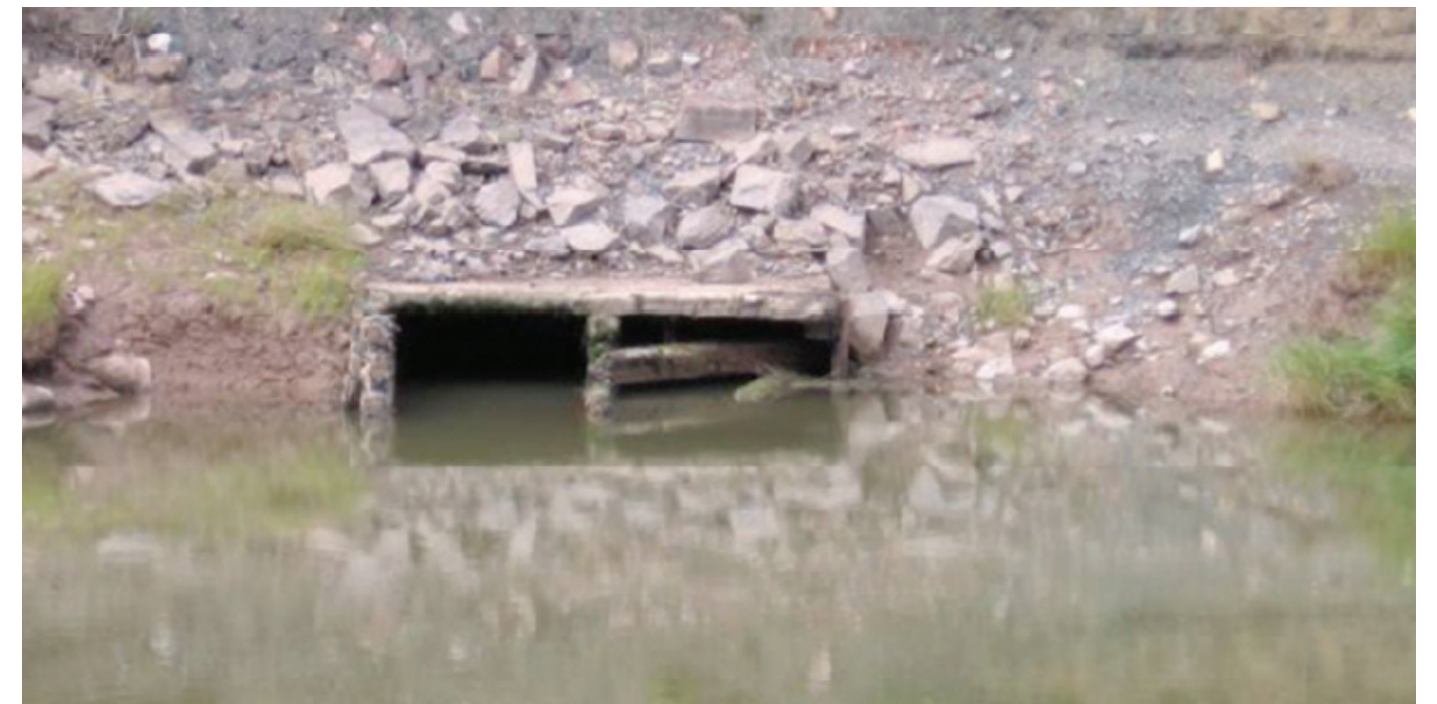
Figure 8. The culvert facilitating tidal exchange for the Cheverie Creek salt marsh prior to restoration. Photo credit: Tony Bowron 2002
